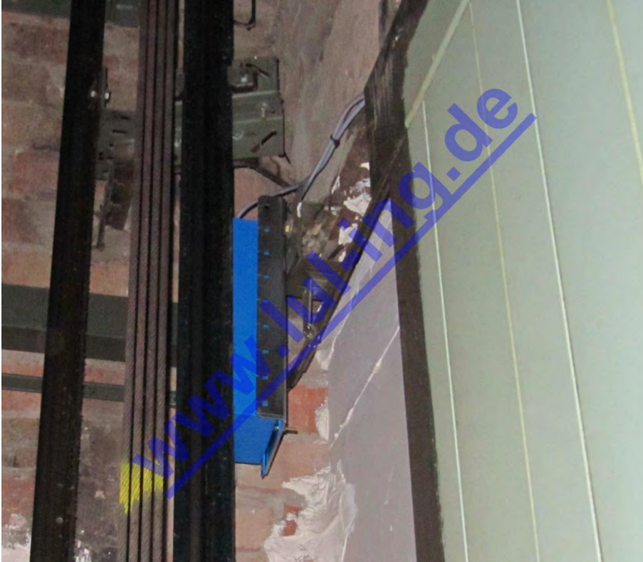
Fig. 7: TSG in Peignen shaft door - fastening for TSG electronics in the shaft
