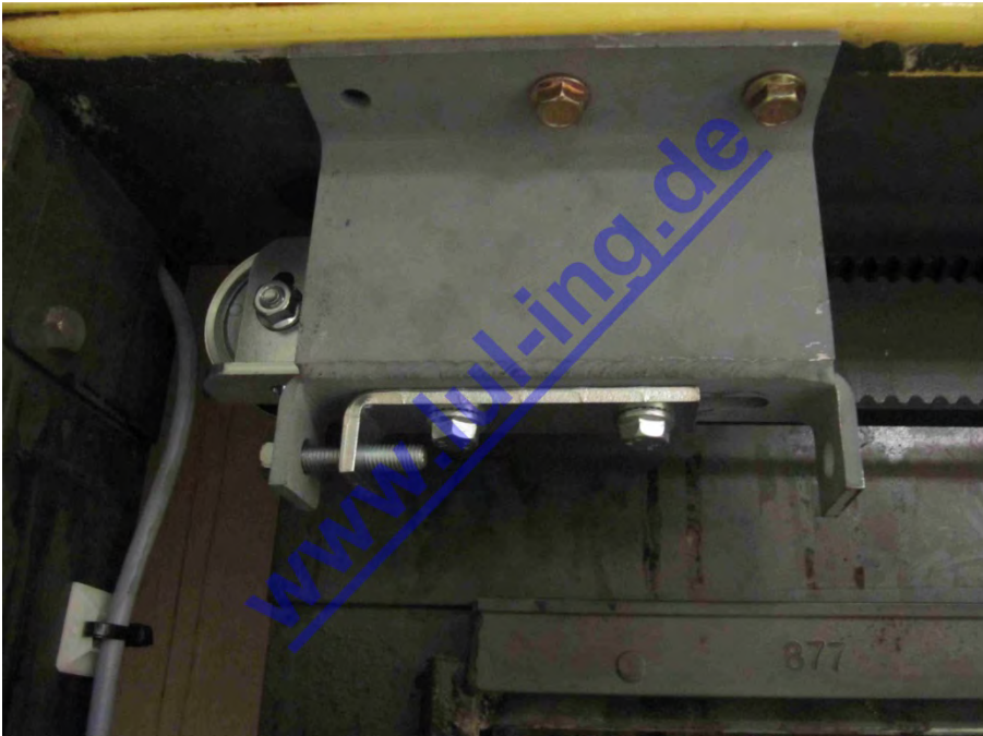
Fig. 5: TSG in Peignen shaft door - counter roller support with clamping station
