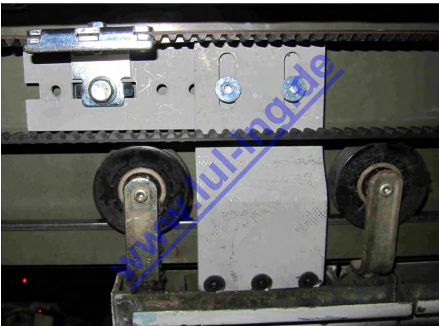
Fig. 6: TSG in Peignen shaft door - door panel carrier
